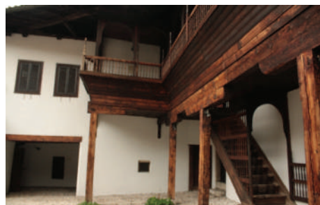
Appendix 12. View of the divhana and pergola located above from the inner courtyard in Svrzo's House
